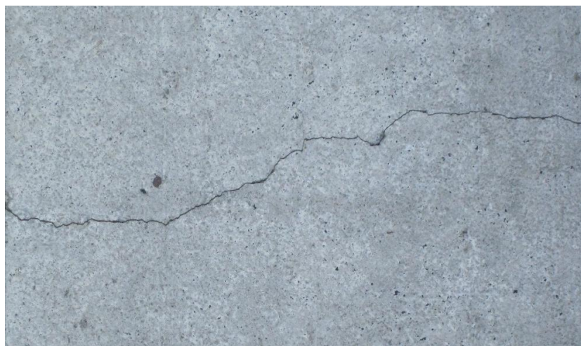
Figure 6. Restrained shrinkage cracking that occurred in a roadside concrete curb; this crack initiated within 56 days of concrete placement; the curb was cured with curing compound.
