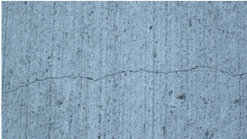
Figure 2. Early-age transverse crack in a concrete pavement slab which widened over time; this crack started within 56 days of concrete placement; the slab was cured using curing compound.
