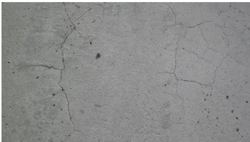
Figure 4. Early-age random cracks that occurred in a concrete floor slab; most of these cracks appeared within 42 days after placing of concrete; the slab was cured using thermal curing blanket.
