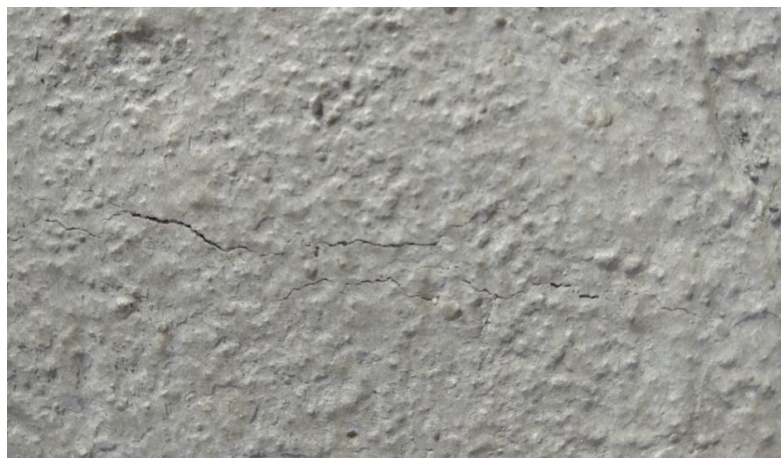
Figure 1. Early-age transverse cracks that occurred in a newly cast reinforced concrete column; these cracks occurred within three days after placing of concrete; the column was cured by wet burlap.
