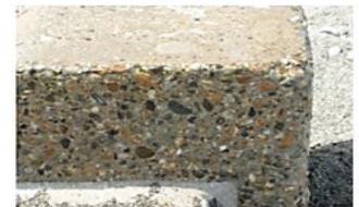
Ordinary Concrete Exposure of aggregate about 40-50%
