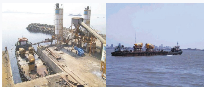
HPC – Bandra-Worli Sea Link Project- Highly flowable concrete with retention time of 5-6 hours (High workability, high retention)
